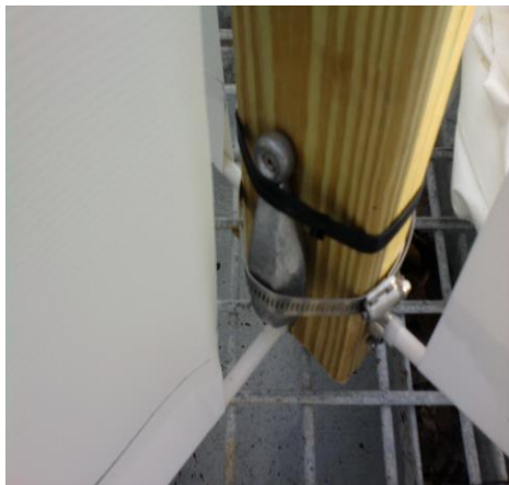
Figure 2a. One option for securing ballast to the bottom of the 2by4
